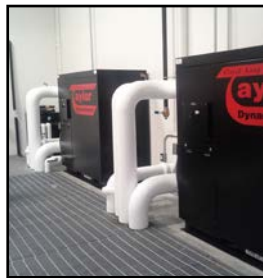
Coolant Storage and Distribution
