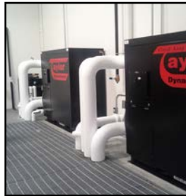
Coolant Storage and Distribution
